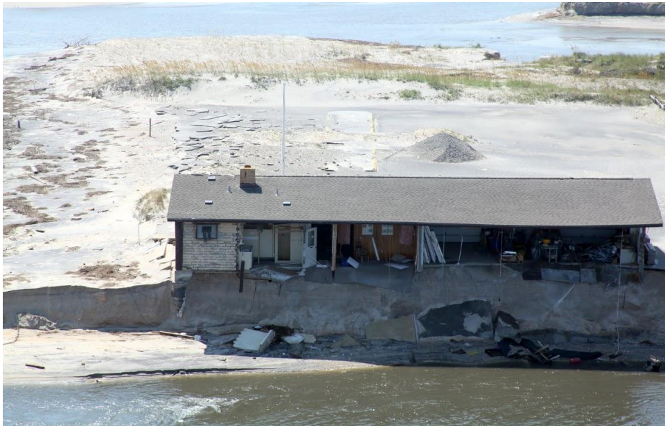
In recent years, natural disasters have added hundreds of millions of dollars to the deferred maintenance backlog. The above photo shows the destruction of a maintenance shop at Pea Island NWR (NC) from Hurricane Irene in 2011.
